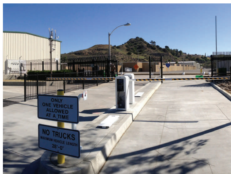
Finishing touches are being made to the new vehicle access gate located next to the Airport Administration Office
